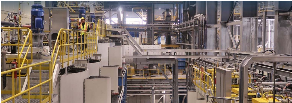
Interior picture of the mill building (shown in the other photos) equipment we previously installed.
